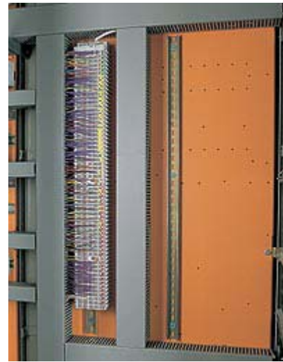
Nr Clearing-up: drilled mounting holes and unused mounting rails demonstrate how the switchgear cabinet was packed out with equipment. Connecting the entire installation can now be done using a fieldbus node equipped with Ethernet controller (see the left side of the picture).
